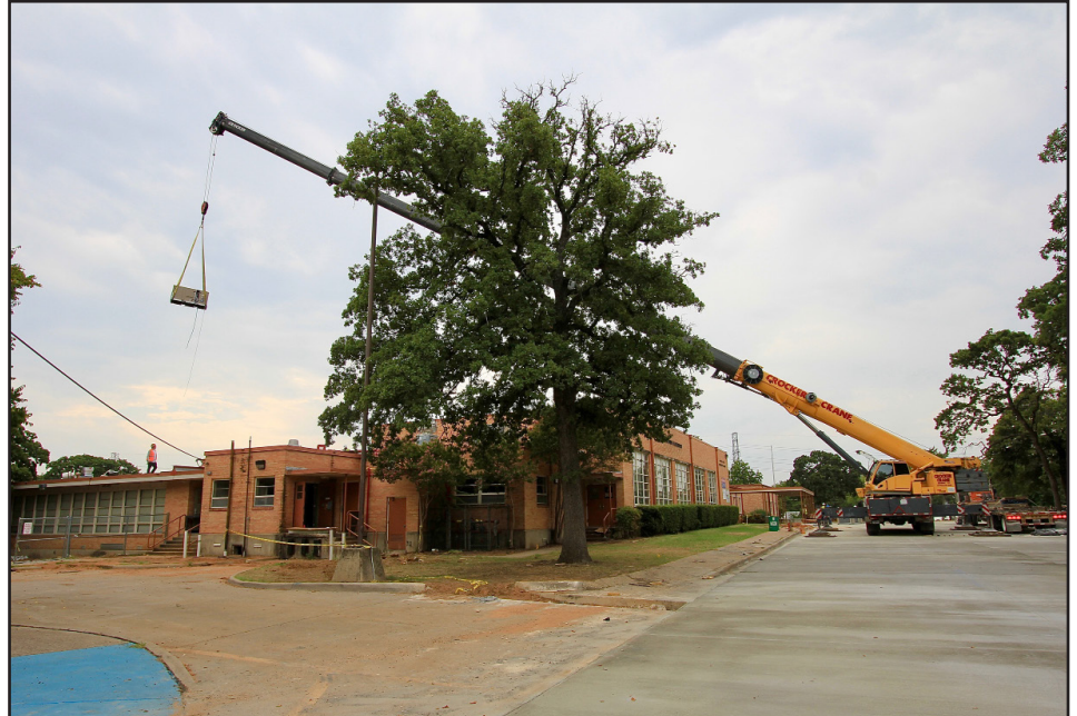
New high-efficiency HVAC units, like this one at South Davis, are part of the bond.
